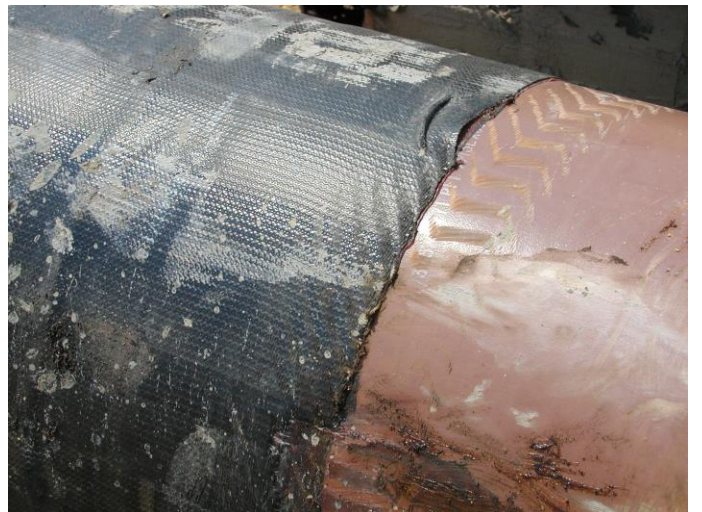
Note damage to main line barrier coating
